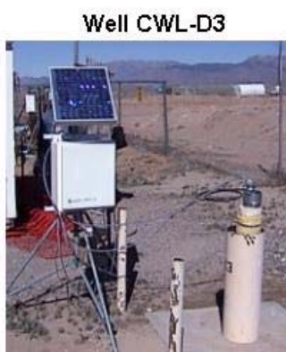
unsaturated-zone well: sensors located ~60 ft below surface
