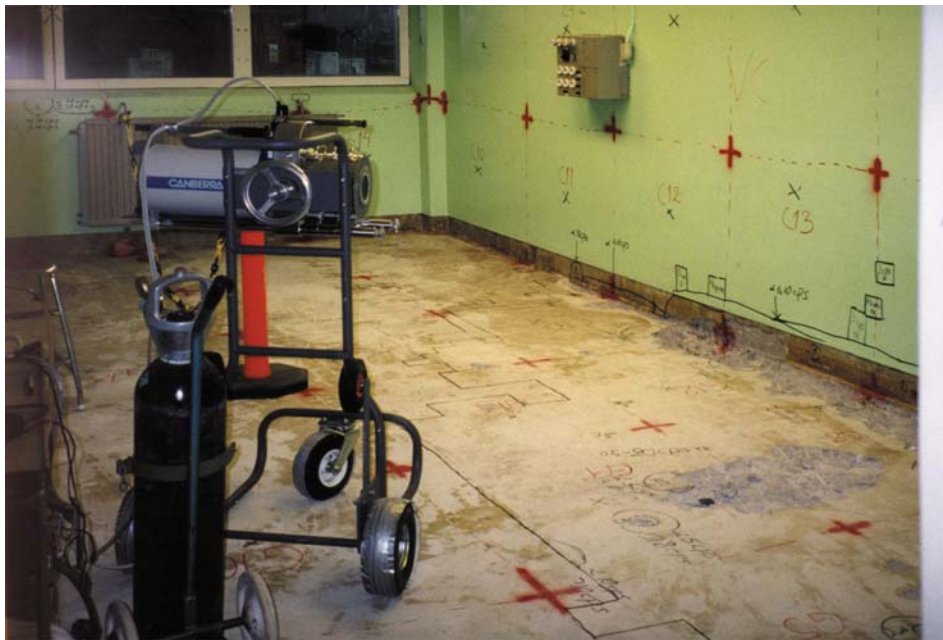
Fig. 3 ISOCS Measurement for clearance.
