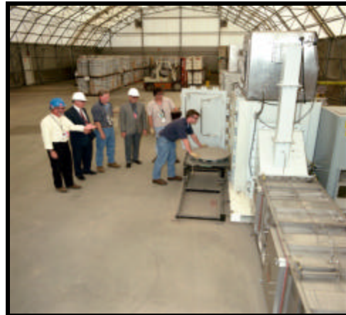
Fig. 6. Drum Vent & Purge System
