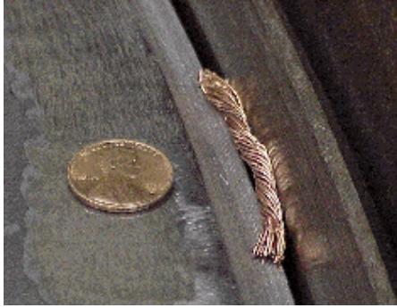
Fig. 2. Copper wire in joint
