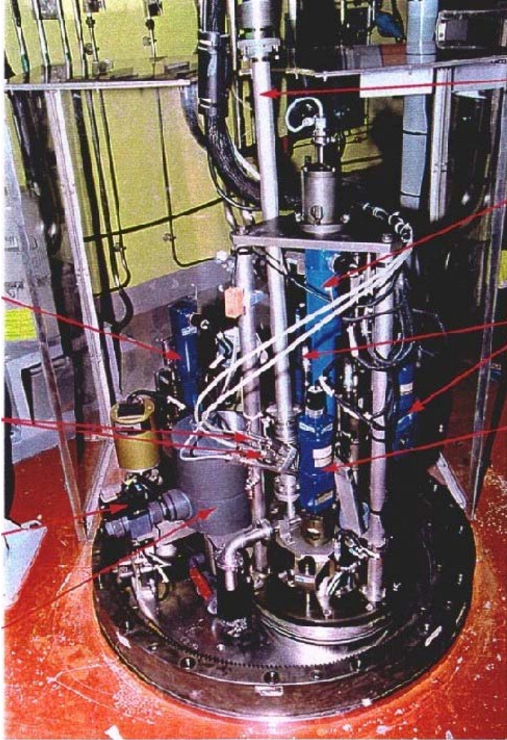
Fig. 2. Automatic Sampling Unit
