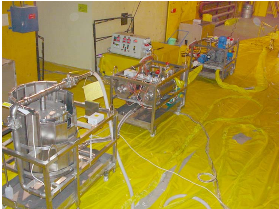
Fig. 4: Portable modular equipment DEZA OD for pre-dismantling chemical circuit decontamination
