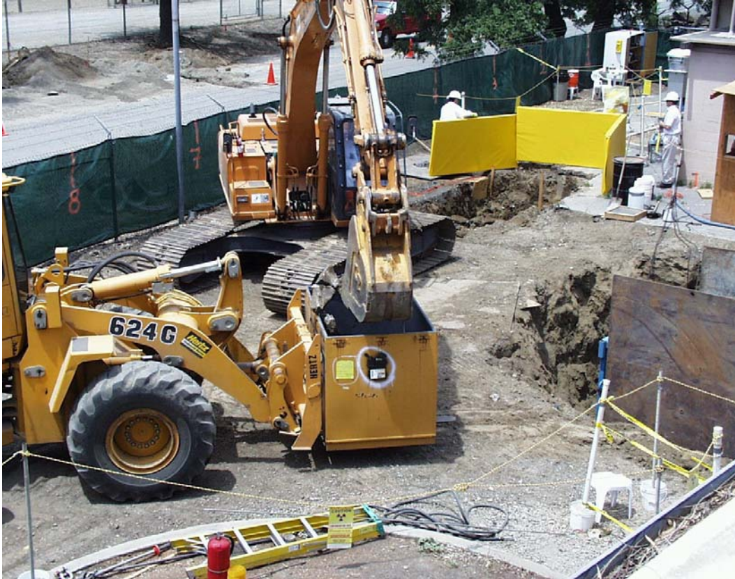
Fig. 2. Loading a Used B-25 Box Using an Excavator and an End Loader
