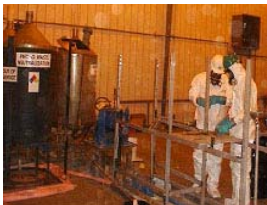
Fig. 1. SEC workers decontaminating a silver recovery unit. Decontamination of scrap metal reduced hazardous waste stream by 200% (2000)
