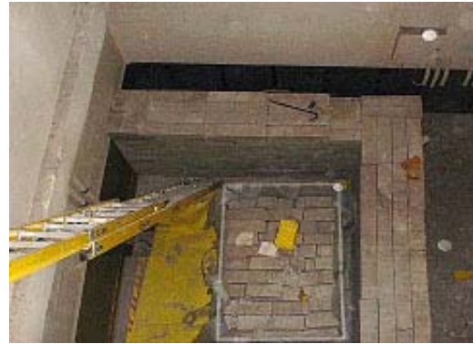
Fig. 3. Segregation of barite shield block. Block was reused, reducing waste volume by 150% (2001)
