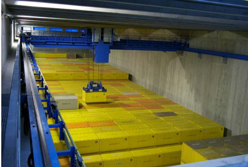
Fig. 2: View of the partially filled storage area C of storage part II
