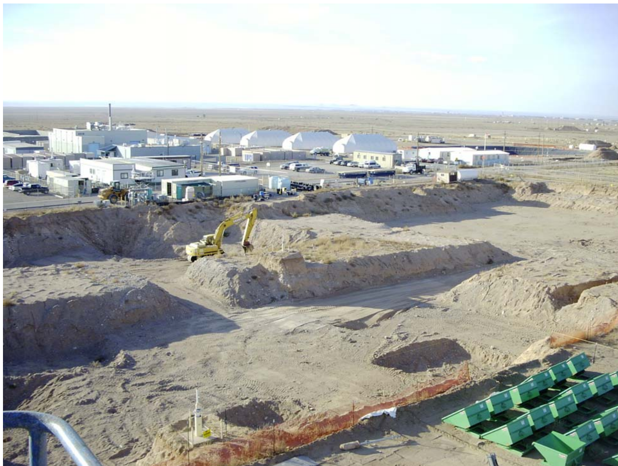
Fig. 1. Excavation of the Buried Debris from the 1.9-acre Chemical Waste Landfill was Completed in June 2001
