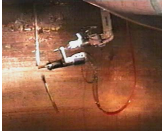
Fig. 2. A hydraulic shear, deployed by the manipulator arm of the Houdini ROV through a tank access riser, successfully cuts a pipe obstructing the landing area of the ROV in this photo captured during operations in tank W-3.
