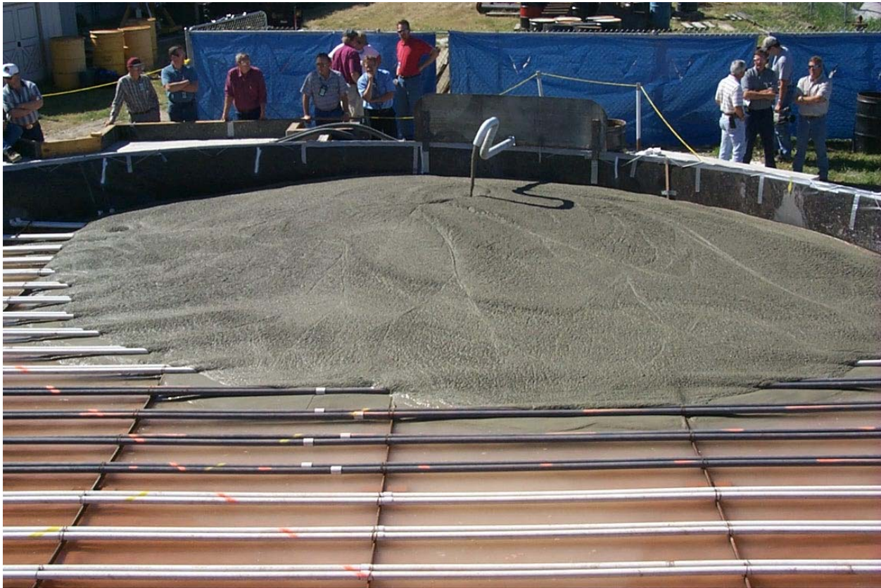
Fig. 3: Pouring grout over the tank bottom to direct fluid to the steam jet entrance
