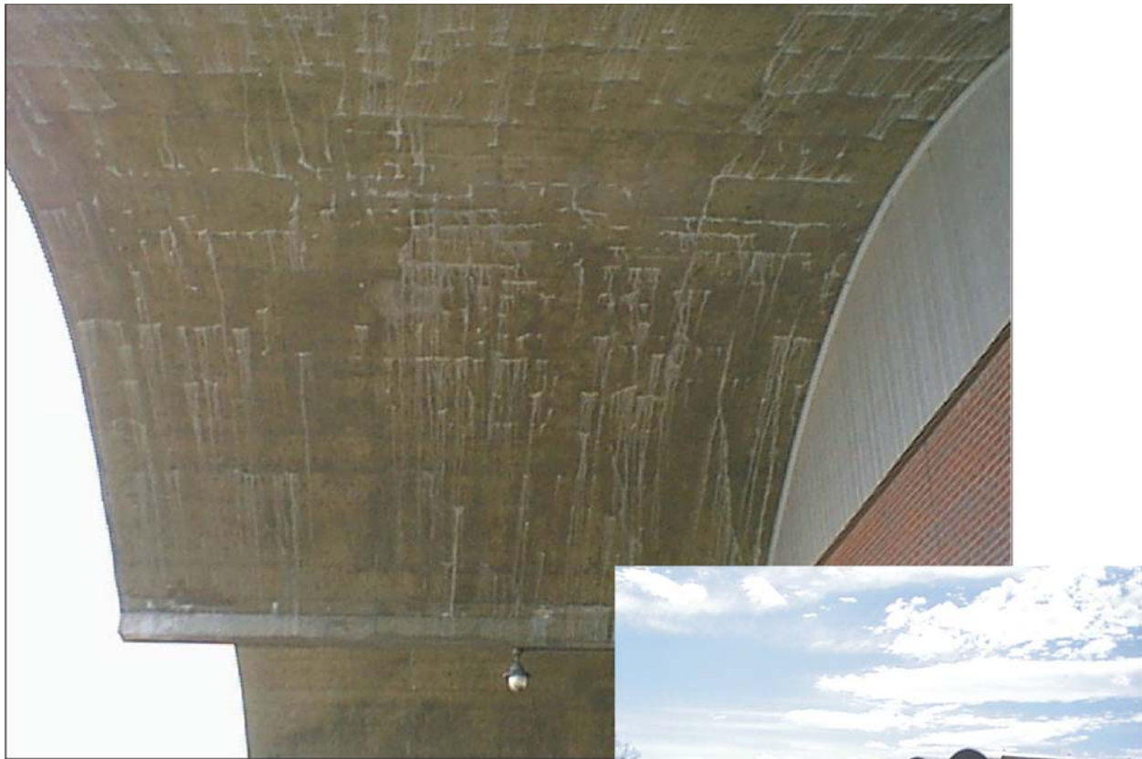
Figure 7. Photograph of building 810 on the Denver Federal Center, Colorado and a close-up of the underside of the roof over the loading dock. Note that water has seeped through along fractures in the concrete, but that rather than dripping, it has flowed along the curvature of the roof.
