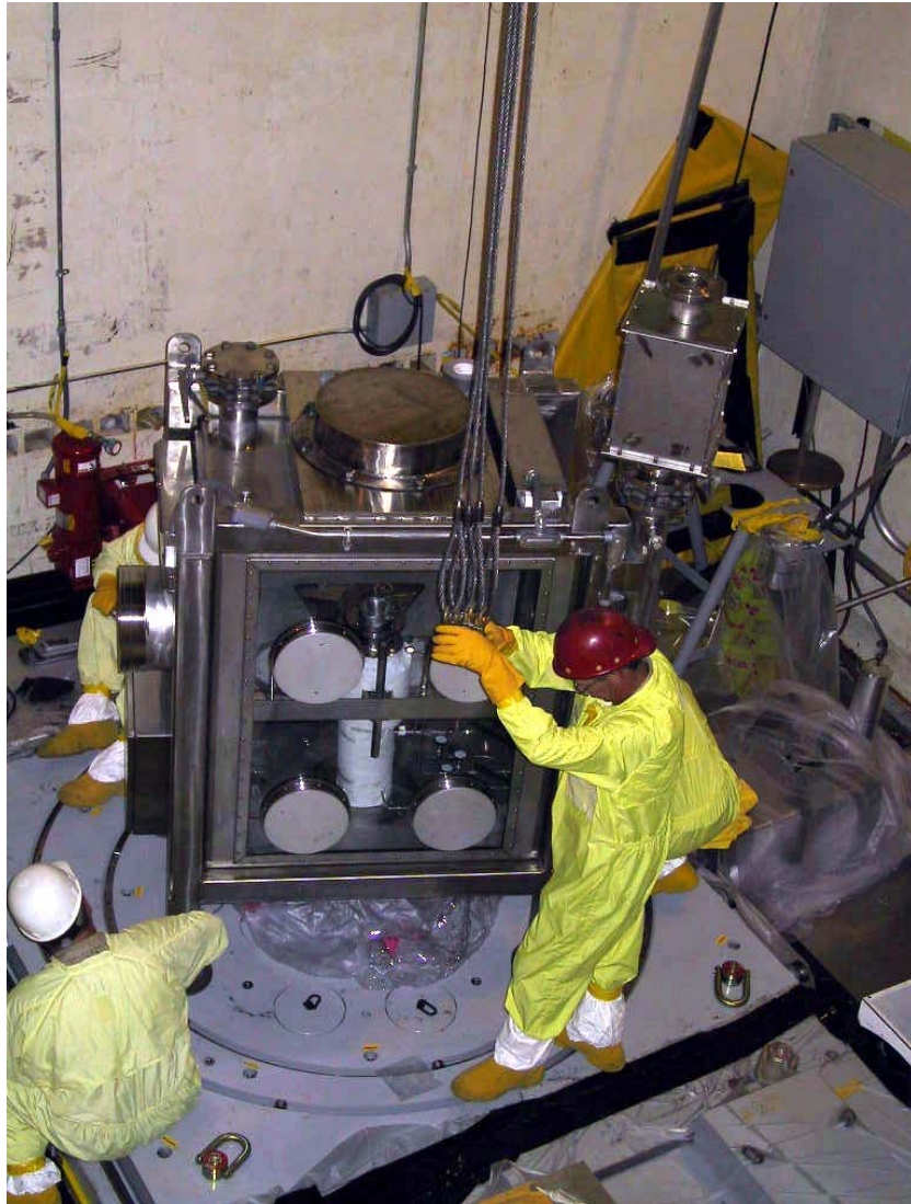
Fig. 4. Salt removal equipment, installation of pool melt probe glove box in the drain tank cell
