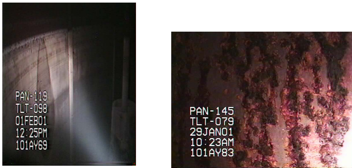
Fig. 2. Interior stain (left) and Annulus Corrosion (right) in DST AY-101.
