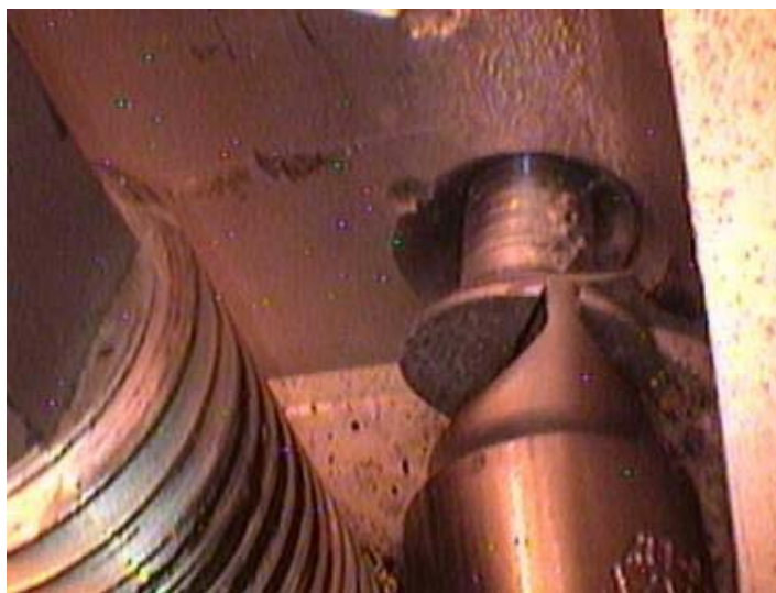
Fig. 2 Unscrewing bolted connections in the region of the reactor core viewed through the video endoscope
