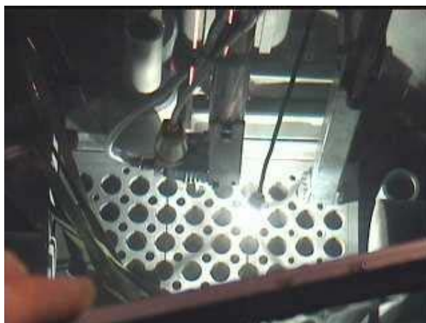
Fig. 3 Cut through the core support plate in the reactor tank using a special underwater saw
