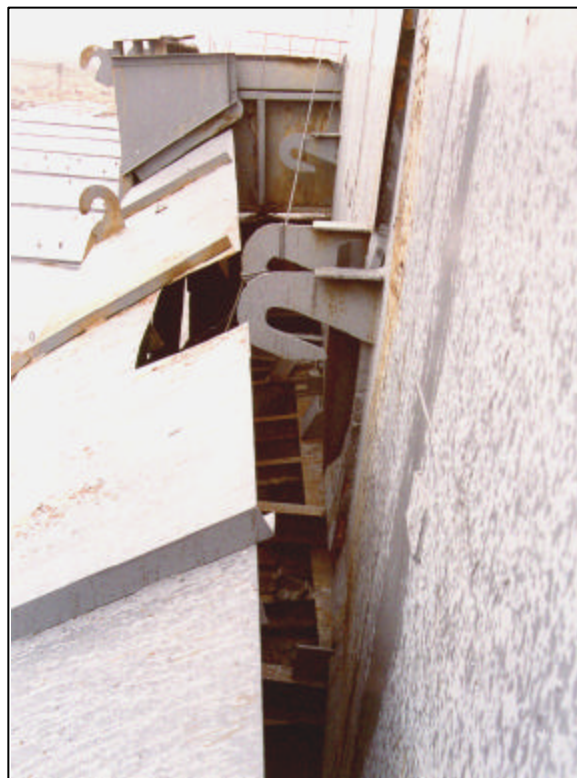
Fig. 1 Shelter Roof Showing Exposures that Allow Rain to Enter
