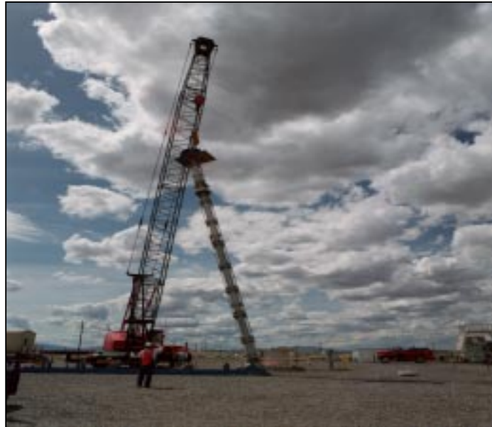
Figure 5. An Example of Tank Farm Long-Length Equipment
