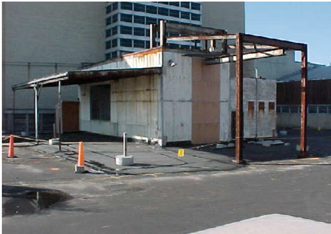
Figure 2 BNL BGRR Canal House structure used for removal of spent fuel and contaminated equipment
