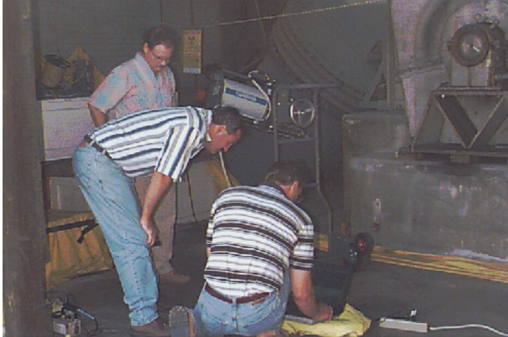
Figure 3 Using in situ ISOCS system to evaluate internal contamination at the BNL BGRR Fan House #5
