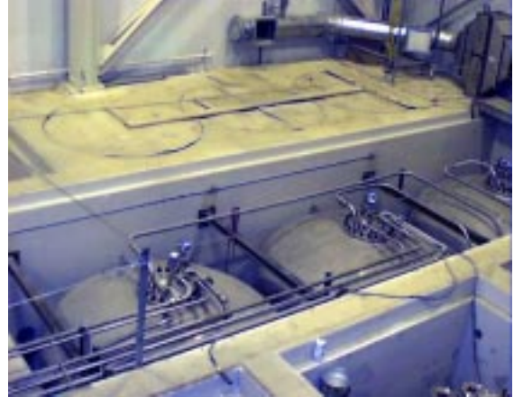
Figure 4 – Slurry Holding Tanks
