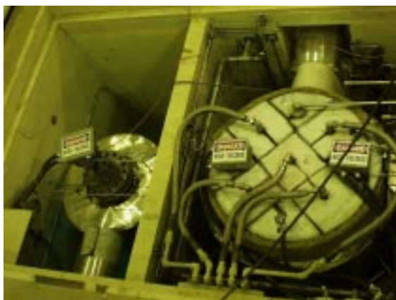
Figure 5 - Process Area - Reformer
