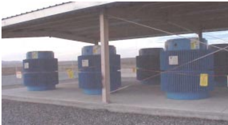
Figure 1 Dry Cask Storage Facility showing concrete pad, CASTOR casks, and metal weather shelter
