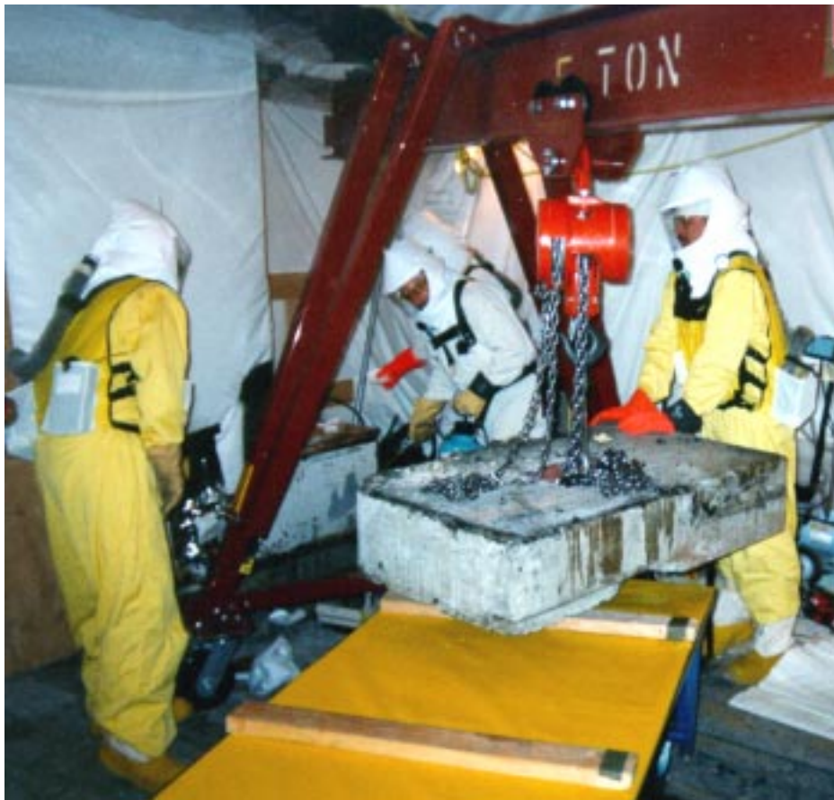
Figure 2. Controlling Hazards. An ERC decommissioning project team uses engineering controls, personal protective equipment, and task-specific work instructions to carefully remove a cover block and access plutonium-contaminated piping.
