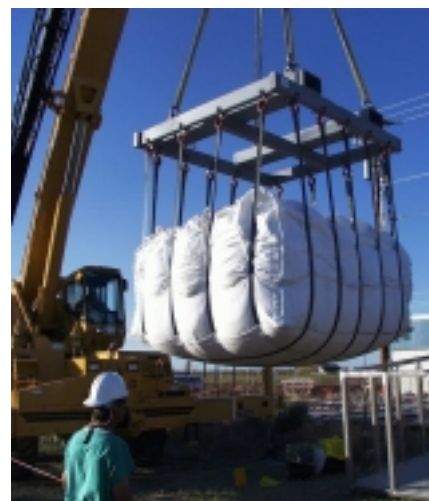
Lifting a full waste container.
