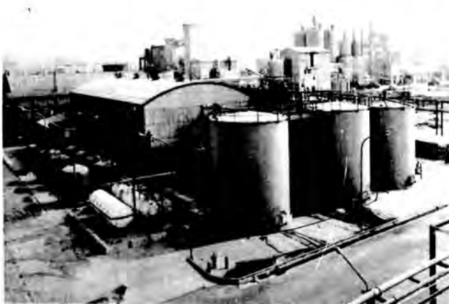
Fig. 2. An over view of URPA plant.
