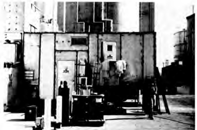
Fig. 6. TVR-III Installed at Palo Verde
