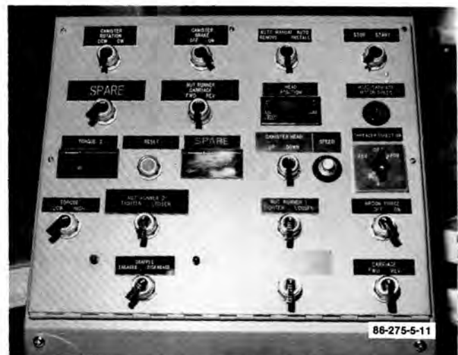
Fig. 7. Control panel of Console.
