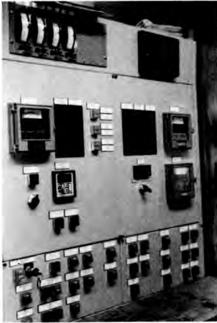
Fig. 4. Section of Control Panel, Note Ease of Reading
