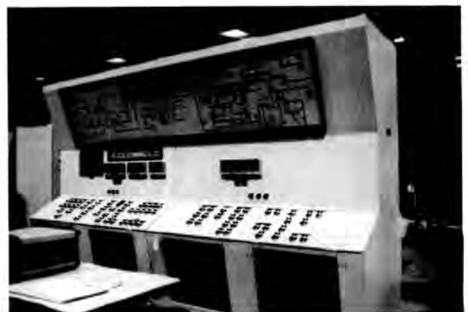
Fig. 10. HF System Control Panel
