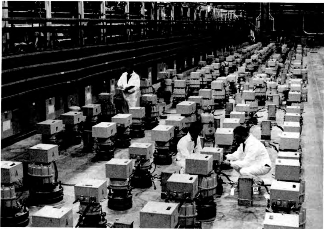
Upper Maintenance area of SIXEP
