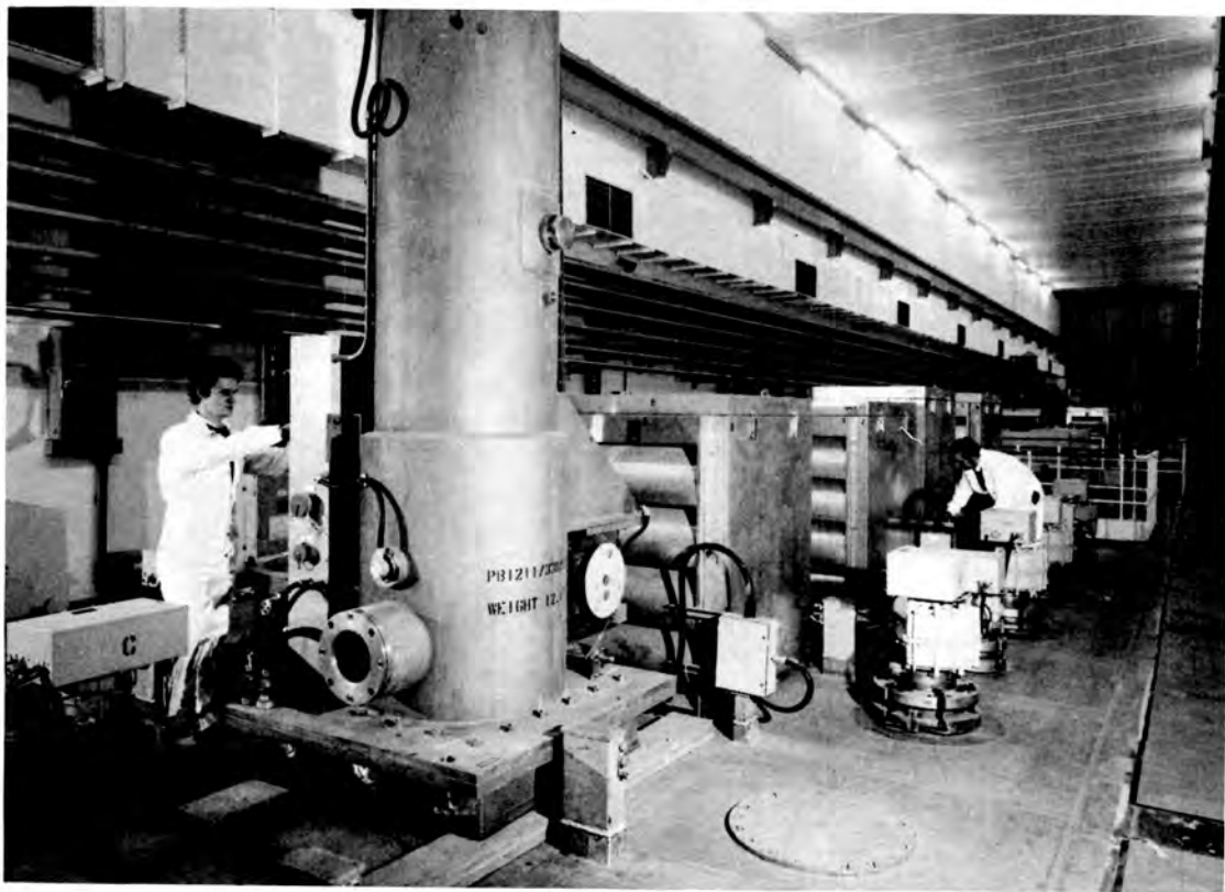
Lower Maintenance Corridor of SIXEP
